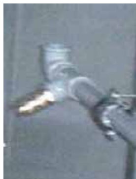
Compressed air installation
