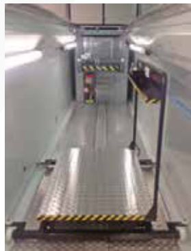
Operator's platform lift
